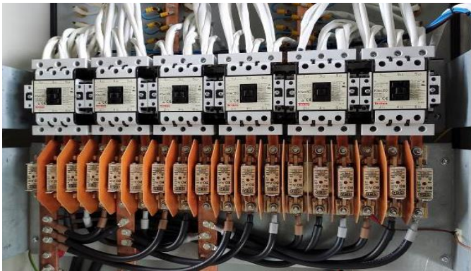
Figure 4. Main 6 contactors with connected set of heating elements
