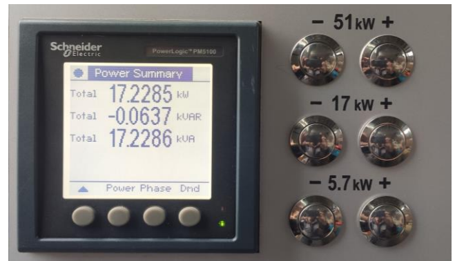
Figure 6. Control panel with power meter PM5110 series.
